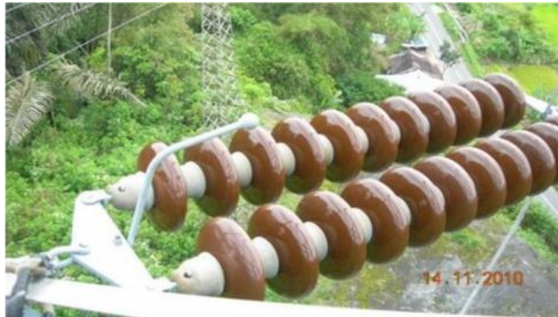
Gambar 2.7 Insulator horizontal string
