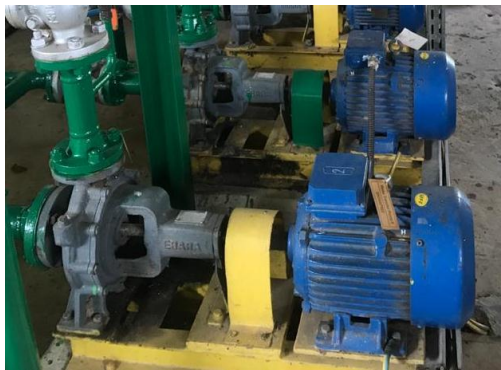
Gambar 2.8 Chemical Dosing Pump (Sumber : PLTG Borang, 2021)
