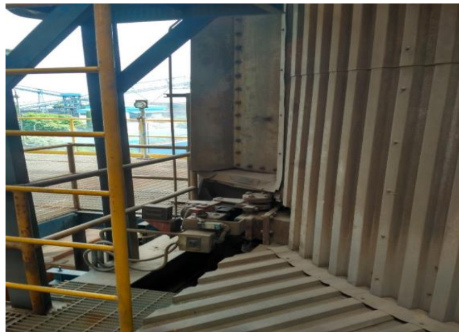
Gambar 2.13 Air Heater Sootblower
