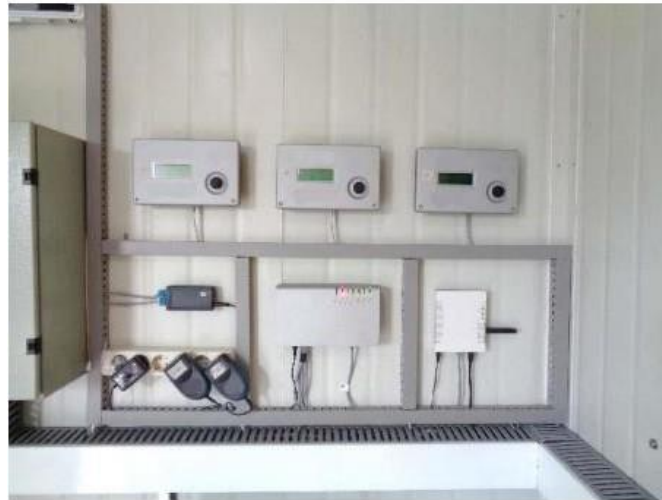
Gambar 2.19 Sistem Monitoring (ii)
