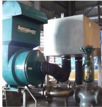
Gambar 2.23 Air/ Oil Separator
