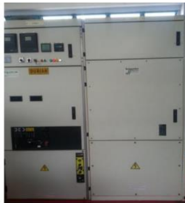
Gambar 2.8 Kubikel Bus Riser / Bus Tie (Interface) di GIS Kotim
