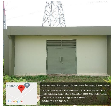
Gambar 2.5 Gardu Tipe Beton
