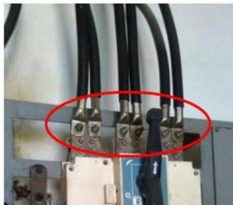
Gambar 2.1 Unit Masukan ( Incoming ) PHB TR
