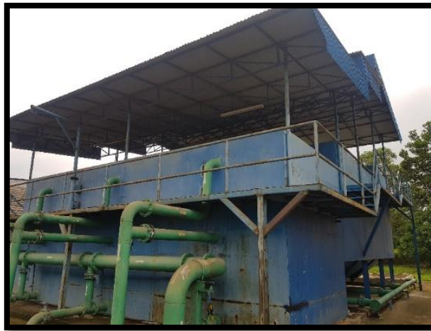
Gambar 2. 2 Water Treatment Plant (Sumber: Dokumentasi Pribadi)
