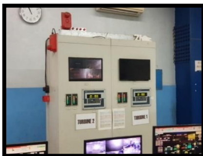
Gambar 2. 31 Governor 505 Turbine Control
