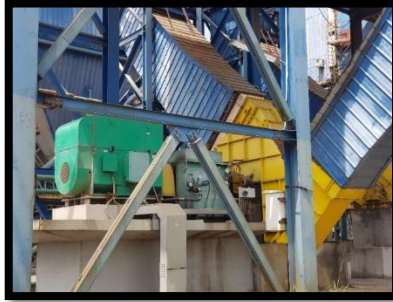
Gambar 2. 24 Induced Draft Fan (Sumber: Dokumentasi Pribadi)
