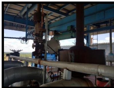
Gambar 2. 28 Steam Blow & Safety Valve (Sumber: Dokumentasi Pribadi)
