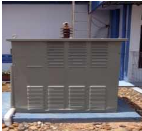
Gambar 2.2 Neutral Grounding Resistance
