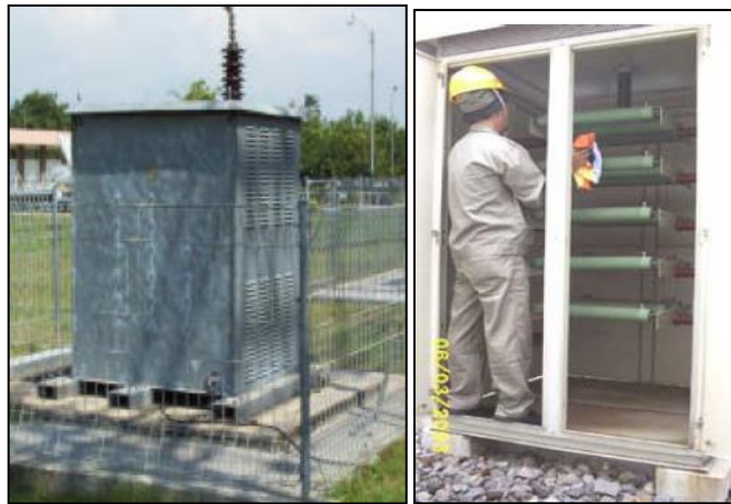
Gambar 2.25 Neutral grounding resistance (NGR)
