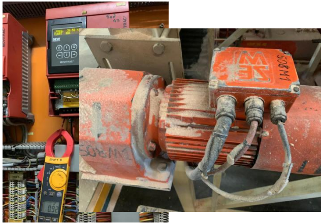
Gambar 2.4.6 Inverter merk SEW Gambar 2.4.7 Motor Conveytor (Sanding area)
