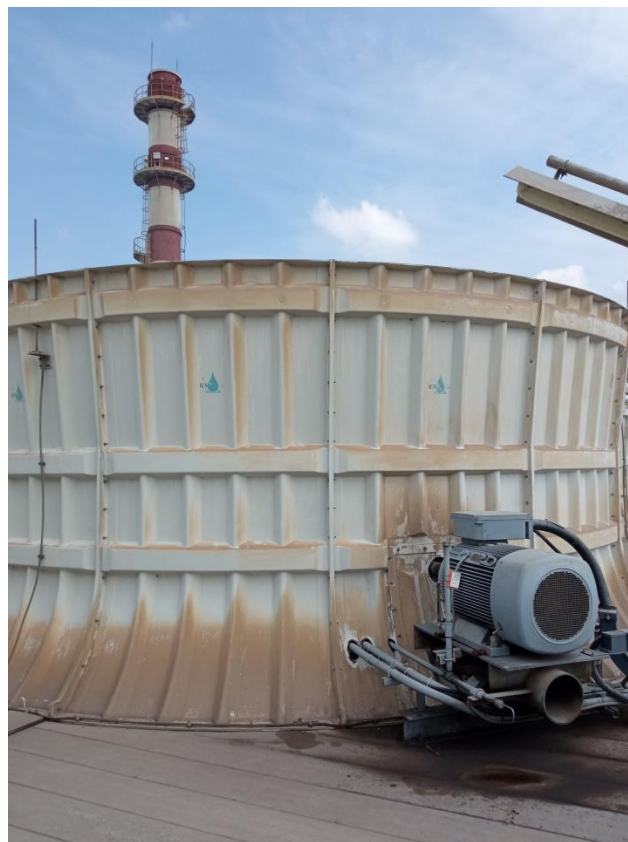
Gambar 2.12 Cooling tower di PT. PLN (Persero) Keramasan Palembang
