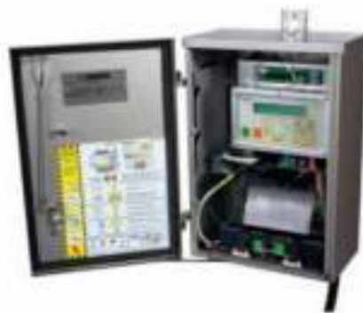
Gambar 2.12 Kubikel / Panel pengendali Load break switch (LBS)
