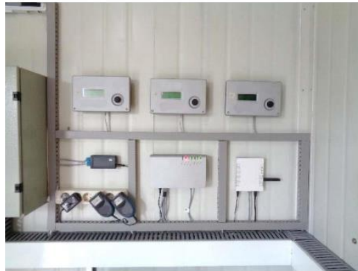
Gambar 2.25 Sistem Monitoring (ii)
