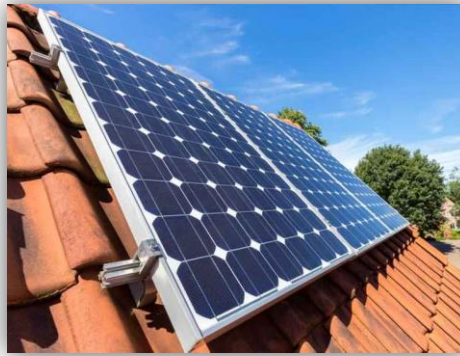
Gambar 2.11 Tampilan Solar Panel
