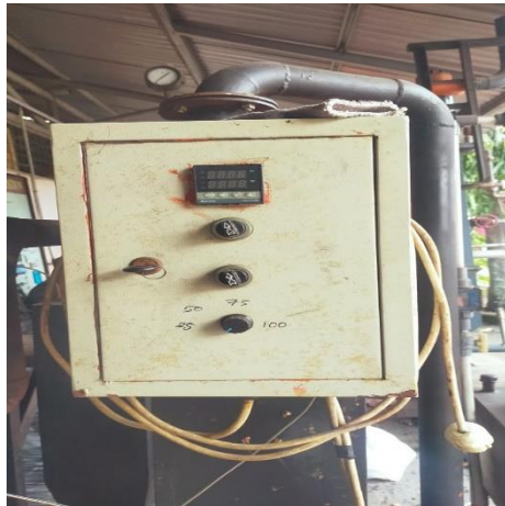
L3.10 Control Panel
