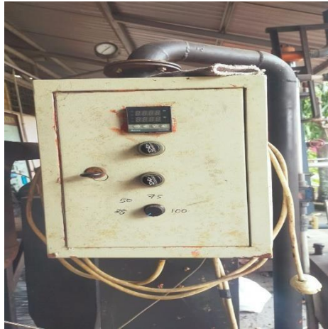
L3.10 Control Panel
