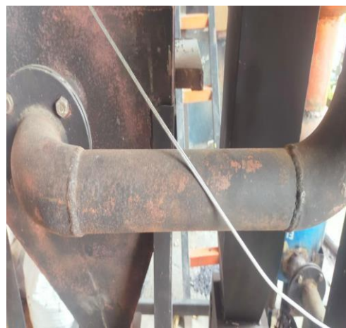
L3.9 Separator Cyclone
