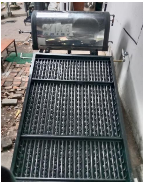
Gambar 18. Solar Water Heater Tampak Atas
