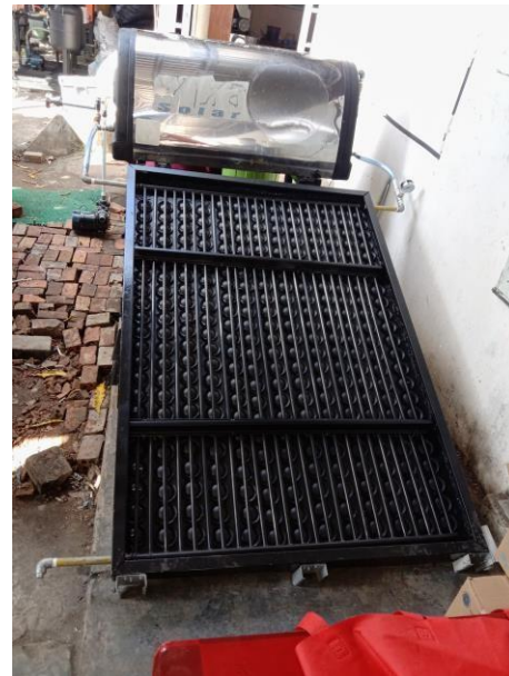
Gambar 20. Solar Water Heater
