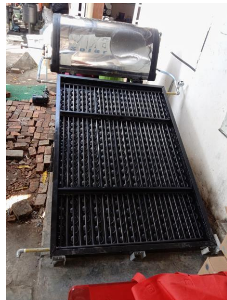
Gambar 5.20. Solar Water Heater
