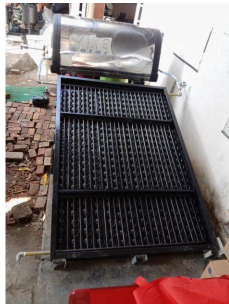
Gambar 20. Solar Water Heater
