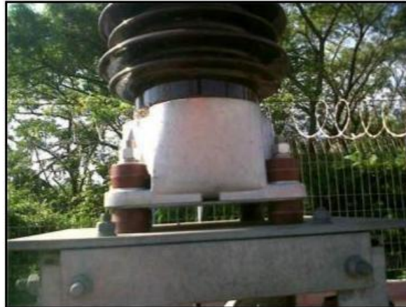
Gambar 2.9 Insulator Lightning Arrester
