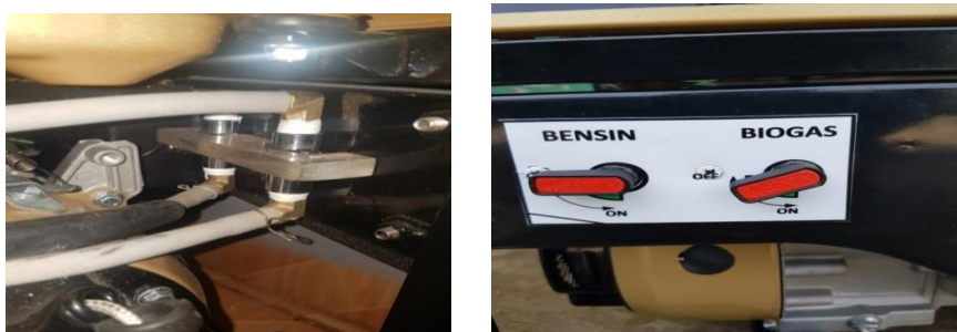
Fig 3. Addition of faucet stock on the generator set
