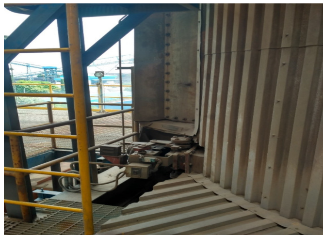
Gambar 2.12 Air Heater Sootblower
