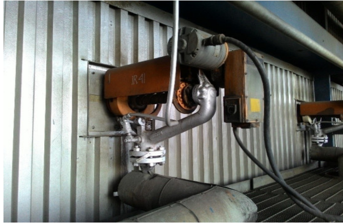
Gambar 2.10 Wall Blower SootBlower
