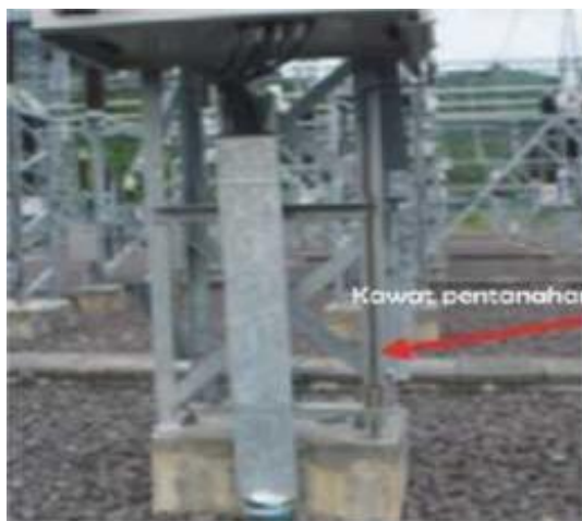
Gambar 2.15 Sistem Pentanahan PMT gas SF6
