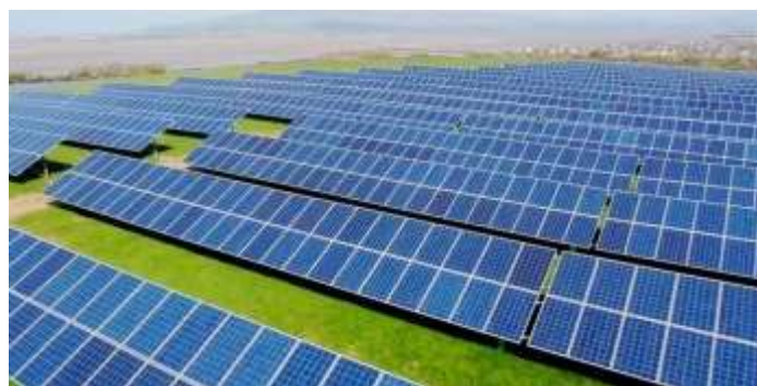
Gambar 2.6 Papan modul solar panel
