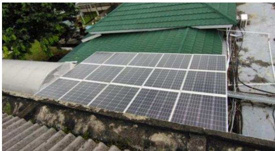
Fig. 9. The projection of monthly production of the On-Grid PV system installed in RSI Siti Khadijah
