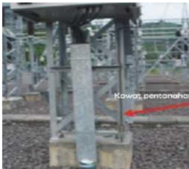
Gambar 2. 18. Sistem Pentanahan PMT gas SF6
