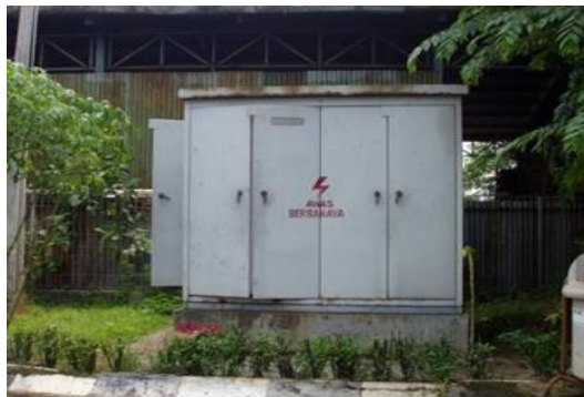
Gambar 2.10 Gardu Metal Clad (MC)
