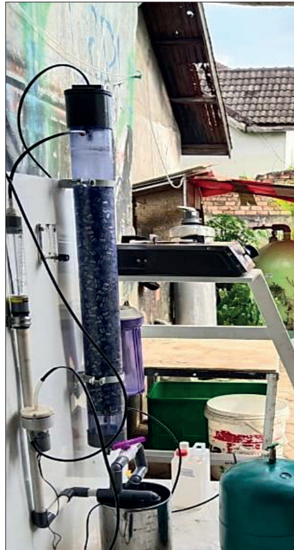
Figure 1. Packed bed scrubber
