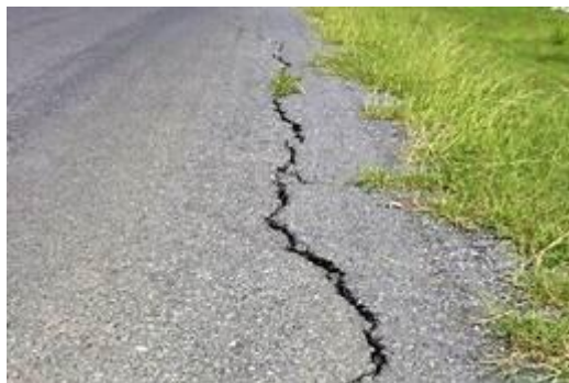
Gambar 2. 9 Edge Joint Crack
