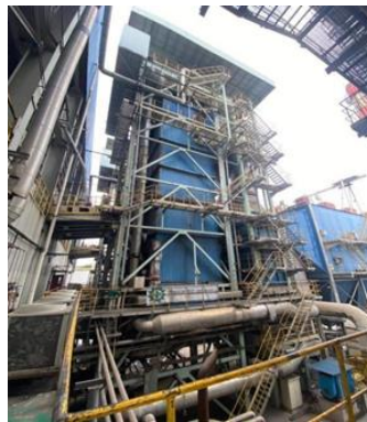
Gambar 2. 2 Boiler Circulating Fluidized Bed (CFB)
