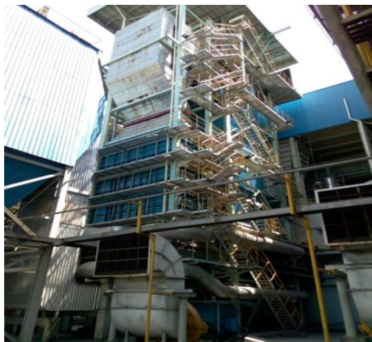
Gambar 2.4 Boiler CFB (PT Bukit Energi Servis Terpadu, 2018)
