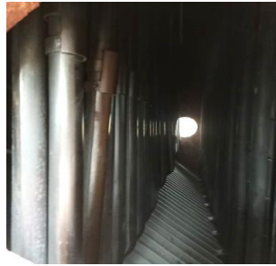
Gambar 2.2 pipa super heater
