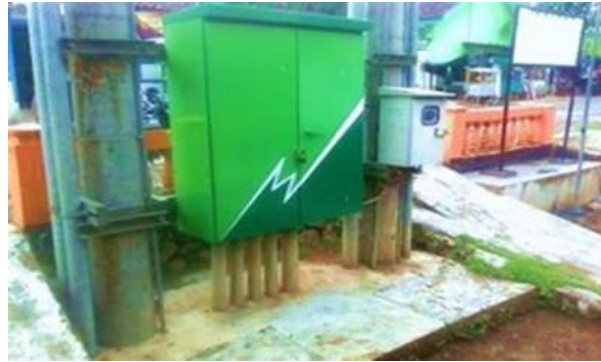
Gambar 2.5 Gardu Tipe Beton
