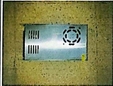
Power supply 12v 5A
