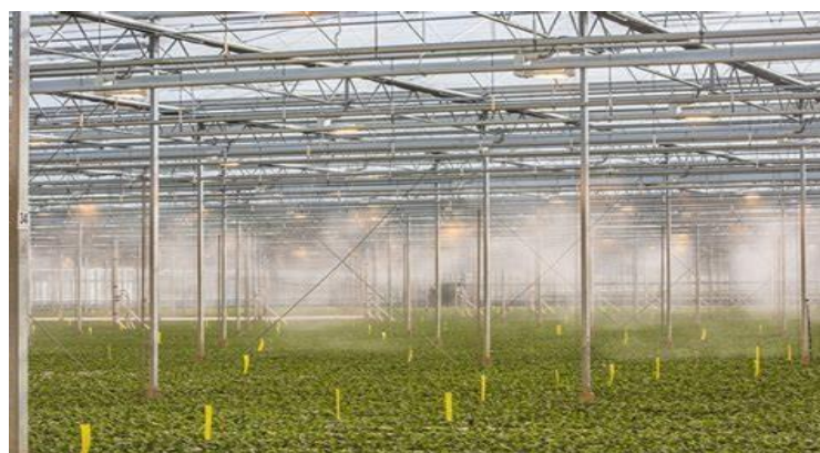
Gambar 2.4 Water Fogging and Cooling System
