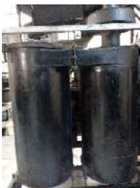
Gas Cooler dan Filter
