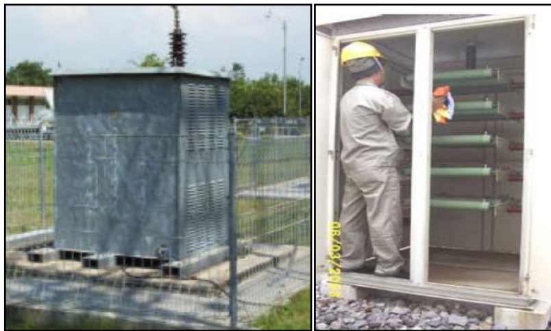
Gambar 2.18 Neutral grounding resistance (NGR)
