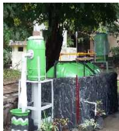
Fixed Dome Digester
