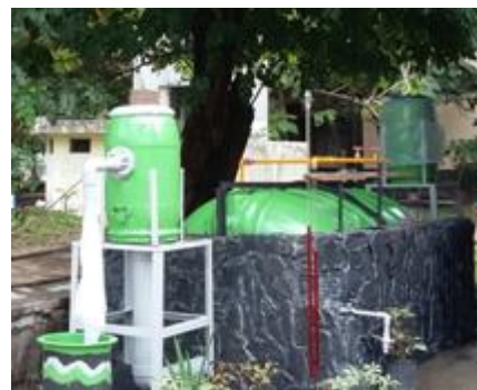
Gambar 25. Fixed Dome Digester
