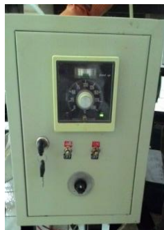
Box Kontrol Panel
