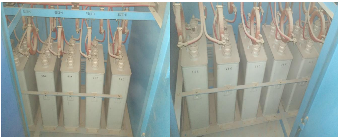
Kapasitor 8 Unit Didalam Panel Kapasitor Bank
