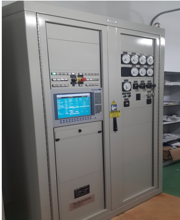
Panel GTG di Room Control Area Sungai Kenawang
