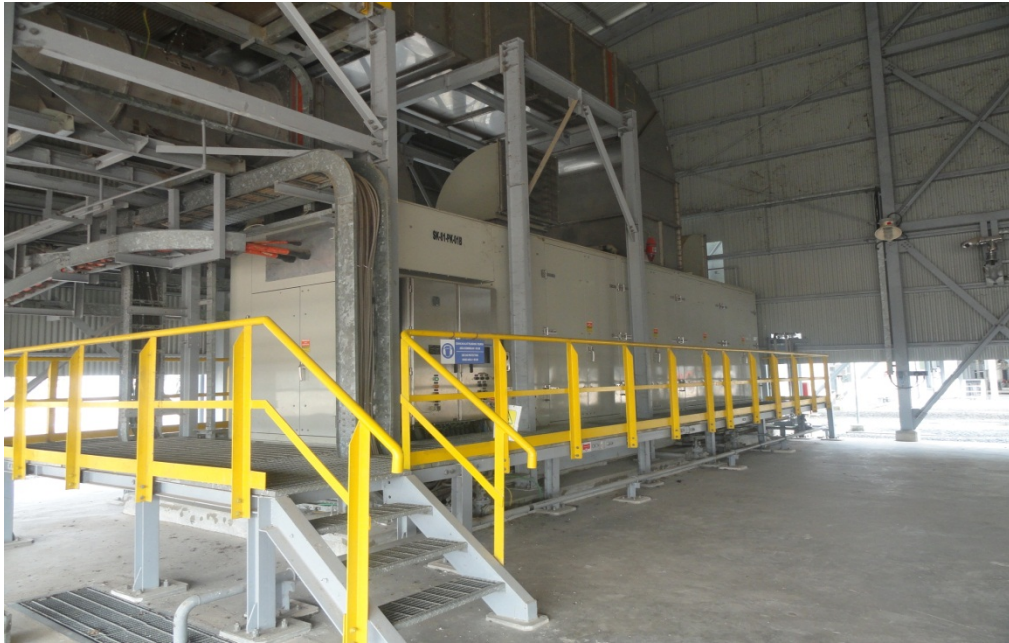
Generator Turbin Gas Taurus 60 di JOB Pertamina-Talisman Jambi Merang
