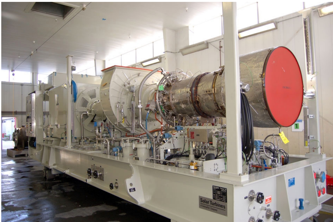
Generator Turbin Gas Engine
