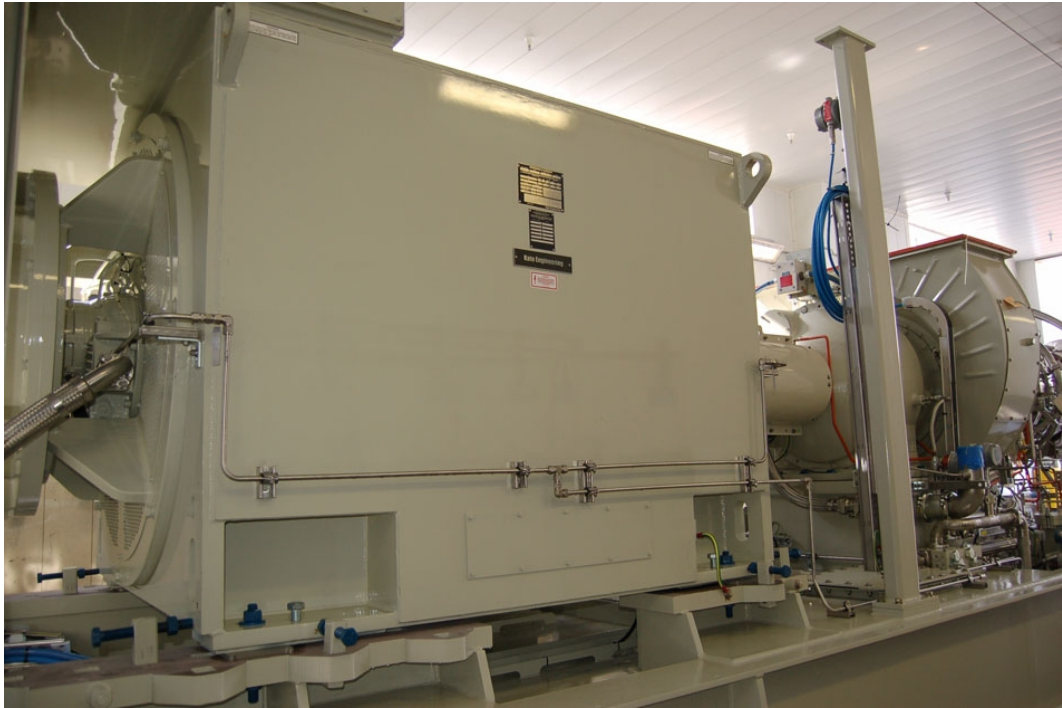
Generator Turbin Gas Engine
