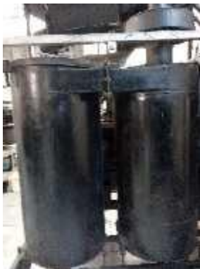
Gas Cooler dan Filter
