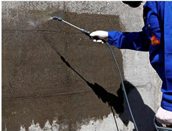
Gambar 10. Penambahan inhibitor korosi
