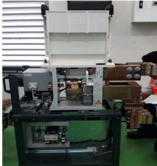
Gambar 2.6 High Speed Circuit Breaker
