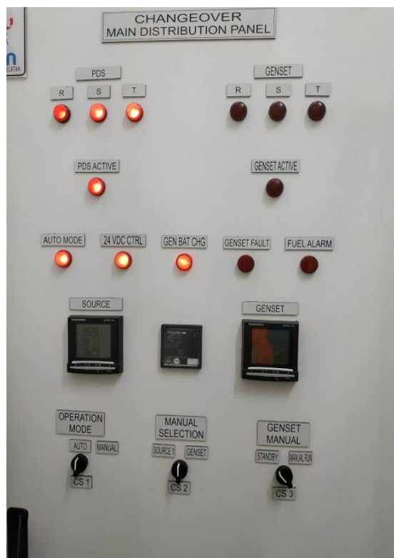
Gambar 2.23 Panel change over switch
