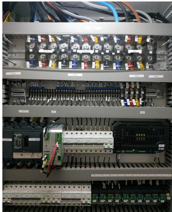
Gambar 2.24 Isi panel change over switch
