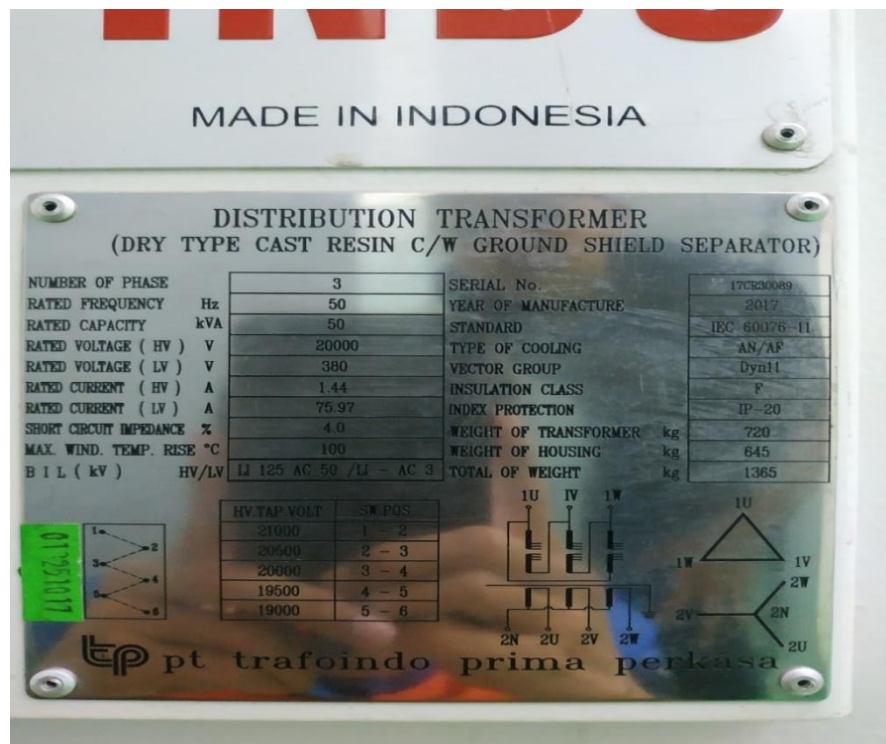
Gambar 2.22 Name Plate Auxiliary Transformator
