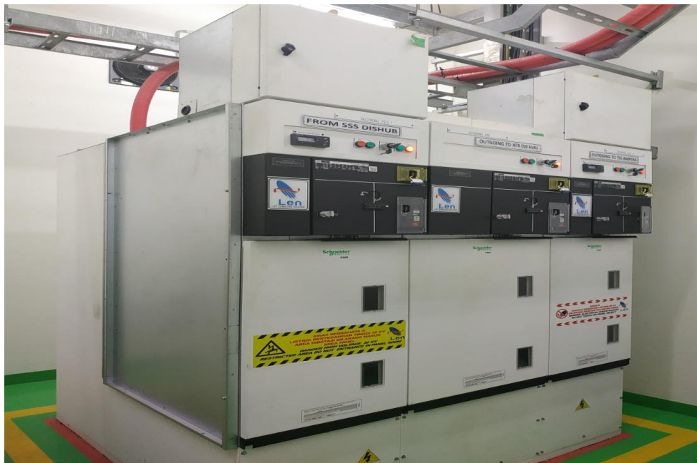
Gambar 2.20 Load Break Switch
