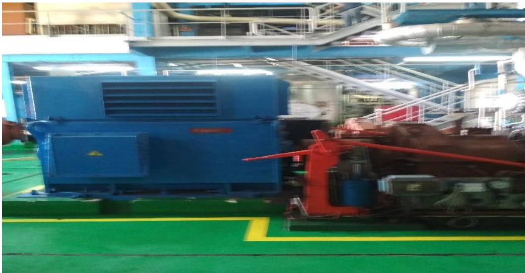
Gambar 2.1 Boiler Feed Water Pump PLTU Bukit Asam
