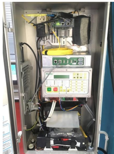
Gambar 2.8 Remote Terminal Unit Recloser Schneider
